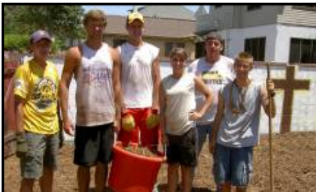
Building a playground area at St. Paul Lutheran Church in Los Angeles, CA
